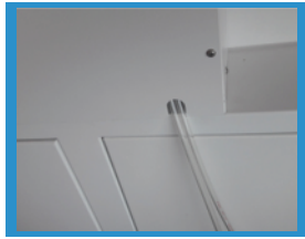
MEDIA COOLING SYSTEM
